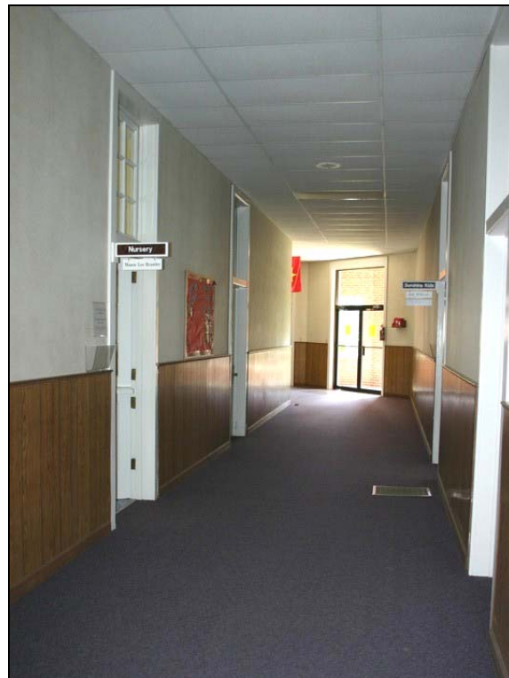
Figure 18: West hall, looking to south entrance, Old Ford School. Penne Sandbeck, NCDOT, October 2010.
