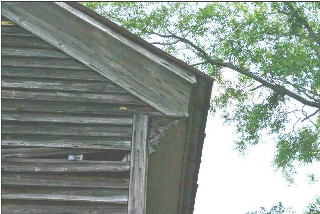
Figure 113: Holliday Store, details of cornerboards, bracket decoration, eaves. Penne Sandbeck, NCDOT, August 2010.
