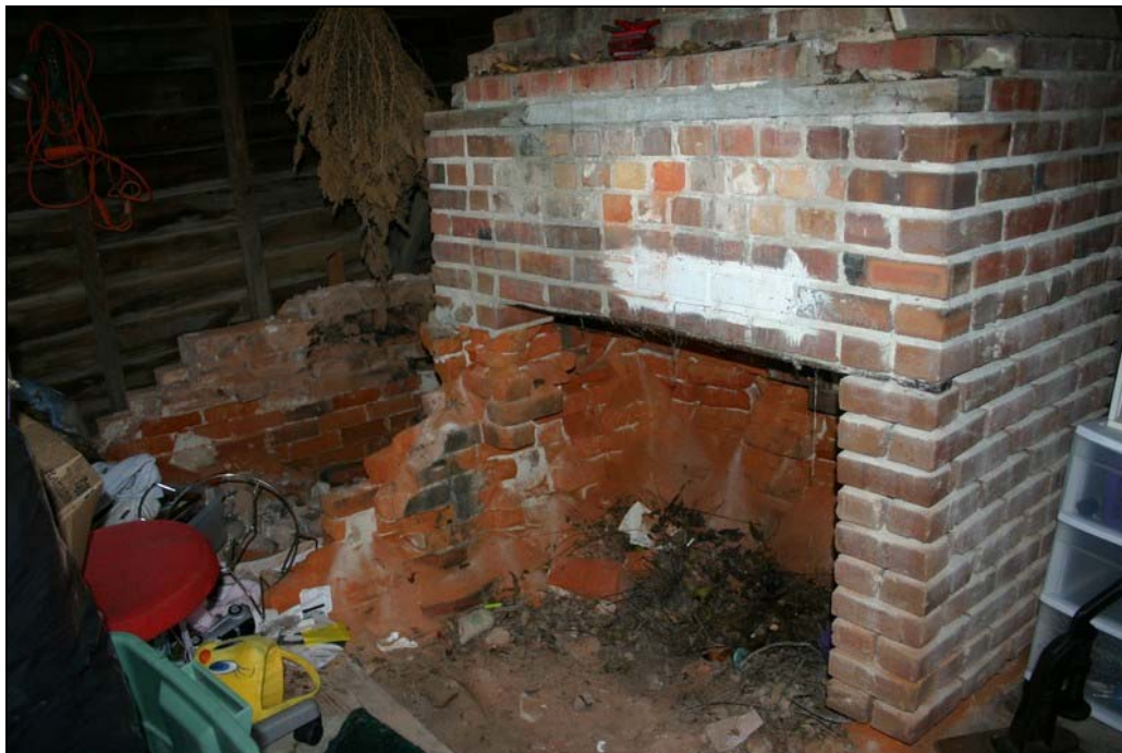
Figure 37: Hearth and former washpit, washhouse at Thad Hodges House. Penne Sandbeck, NCDOT, October 2010.
