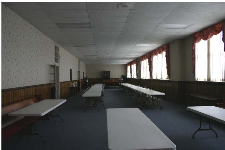
Figure 25: Classroom interiors. One of the most substantial alterations at Old Ford School was removing two classroom partition walls for this common room at the front wing's west central bay. Penne Sandbeck, NCDOT, October 2010.
