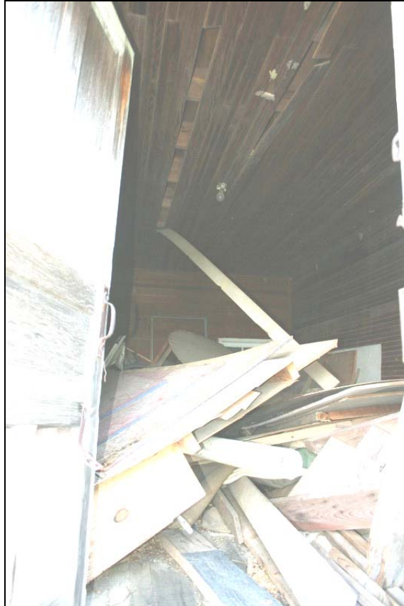
Figure 116: Interior, Holliday Store (door was wide open, no entry was attempted). Penne Sandbeck, NCDOT, August 2010.
