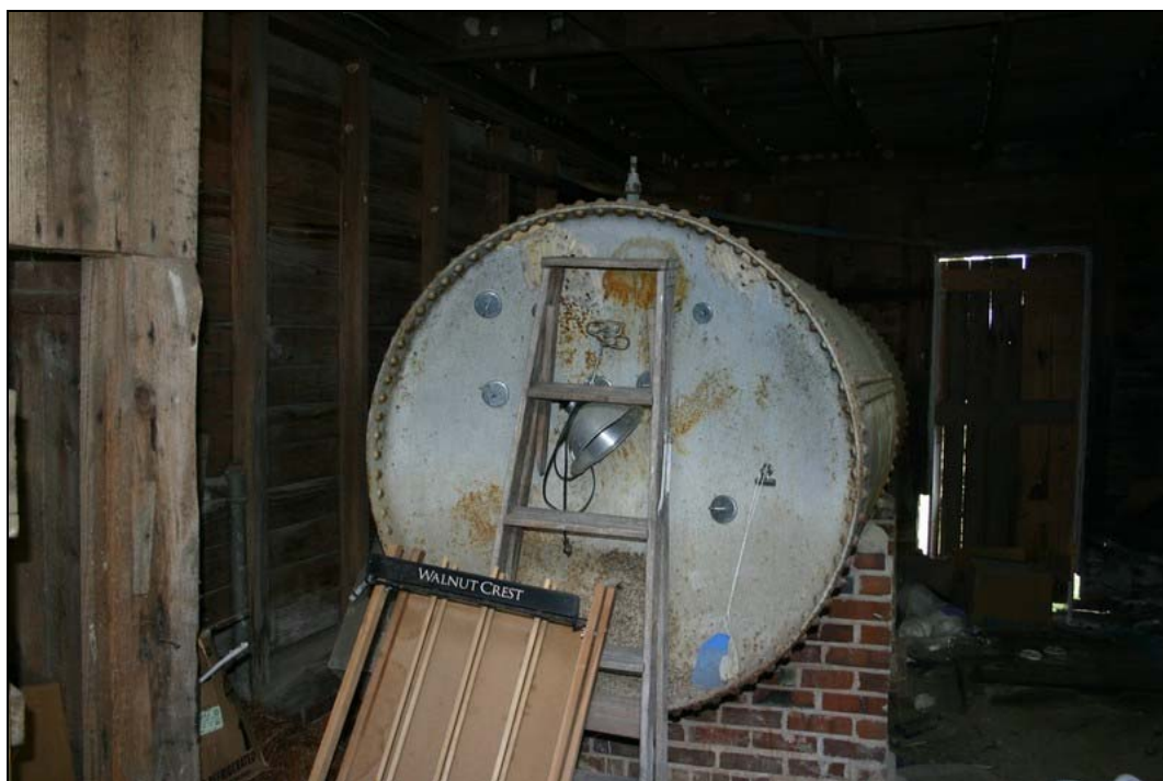
Figure 40: Front of pumphouse tank, boiler pressure gauge (finial at top) still in place. Penne Sandbeck, NCDOT, October 2010.
