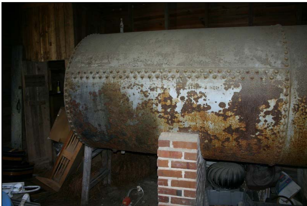
Figure 39: Boiler tank for pumphouse with large rivets from the early twentieth century. Penne Sandbeck, NCDOT, October 2010.
